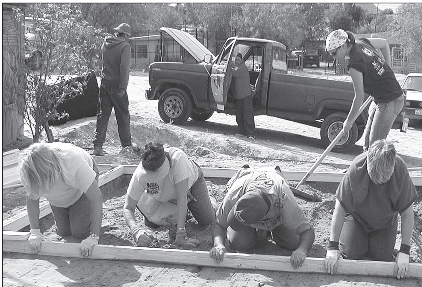
MISSION TEAM MEMBERS (above) worked to level the building site before the concrete foundation could be poured for the house they were building for a Mexican family.
