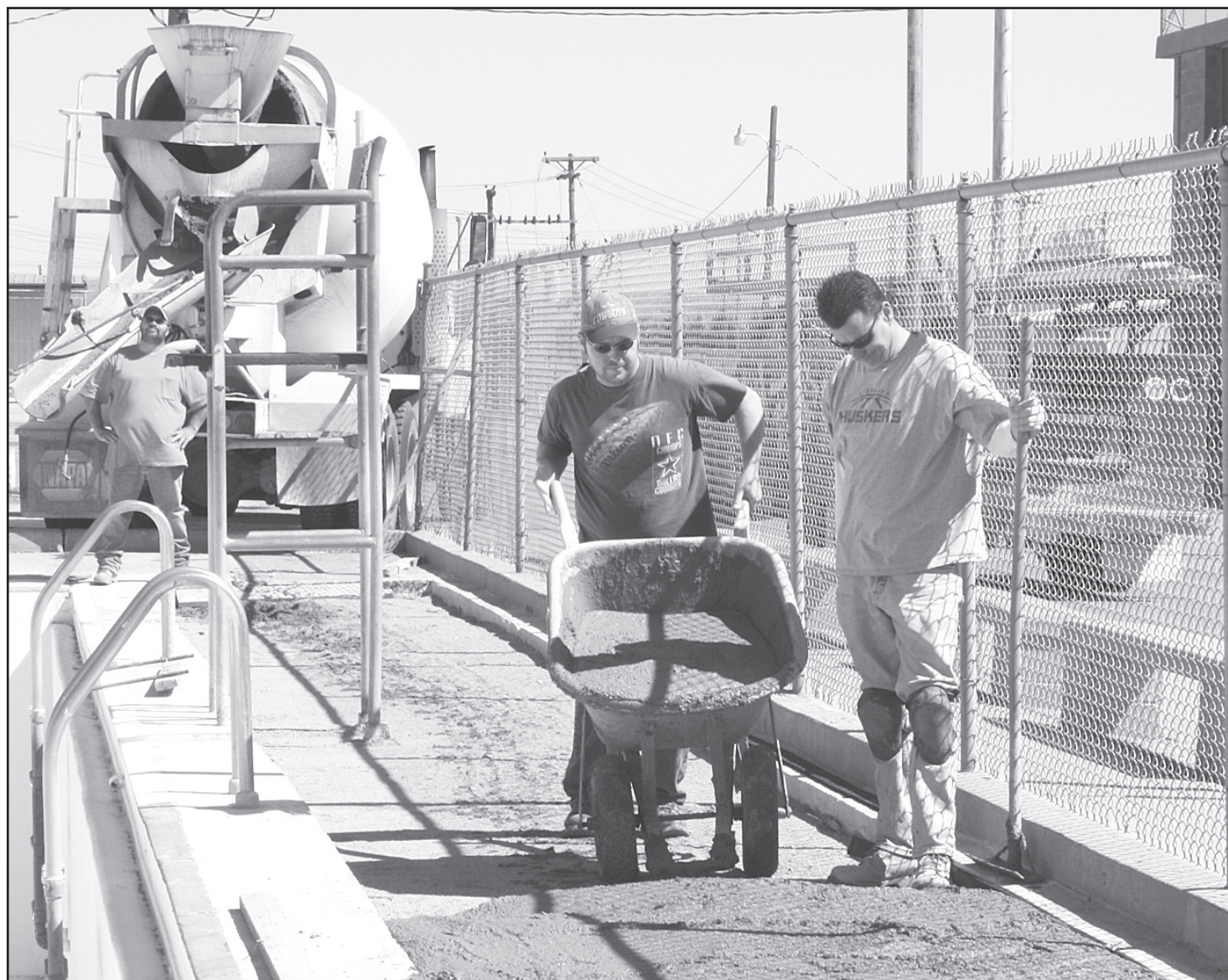
AT THE SWIMMING POOL on Monday afternoon the south side one wheel barrow at a time. Wayne Hackney and crew poured concrete for decking on — Herald staff photo by Kimberly Davis
