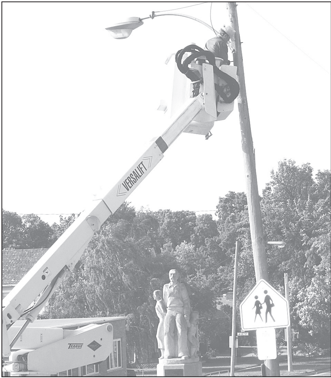
IN THE LINE TRUCK , City Foreman Dan Castle worked on an electric line on north Main Street on Friday after a tree limb knocked it down. A crew trimmed trees along the street that were near the line the same morning. — Herald staff photo by Kimberly Davis
