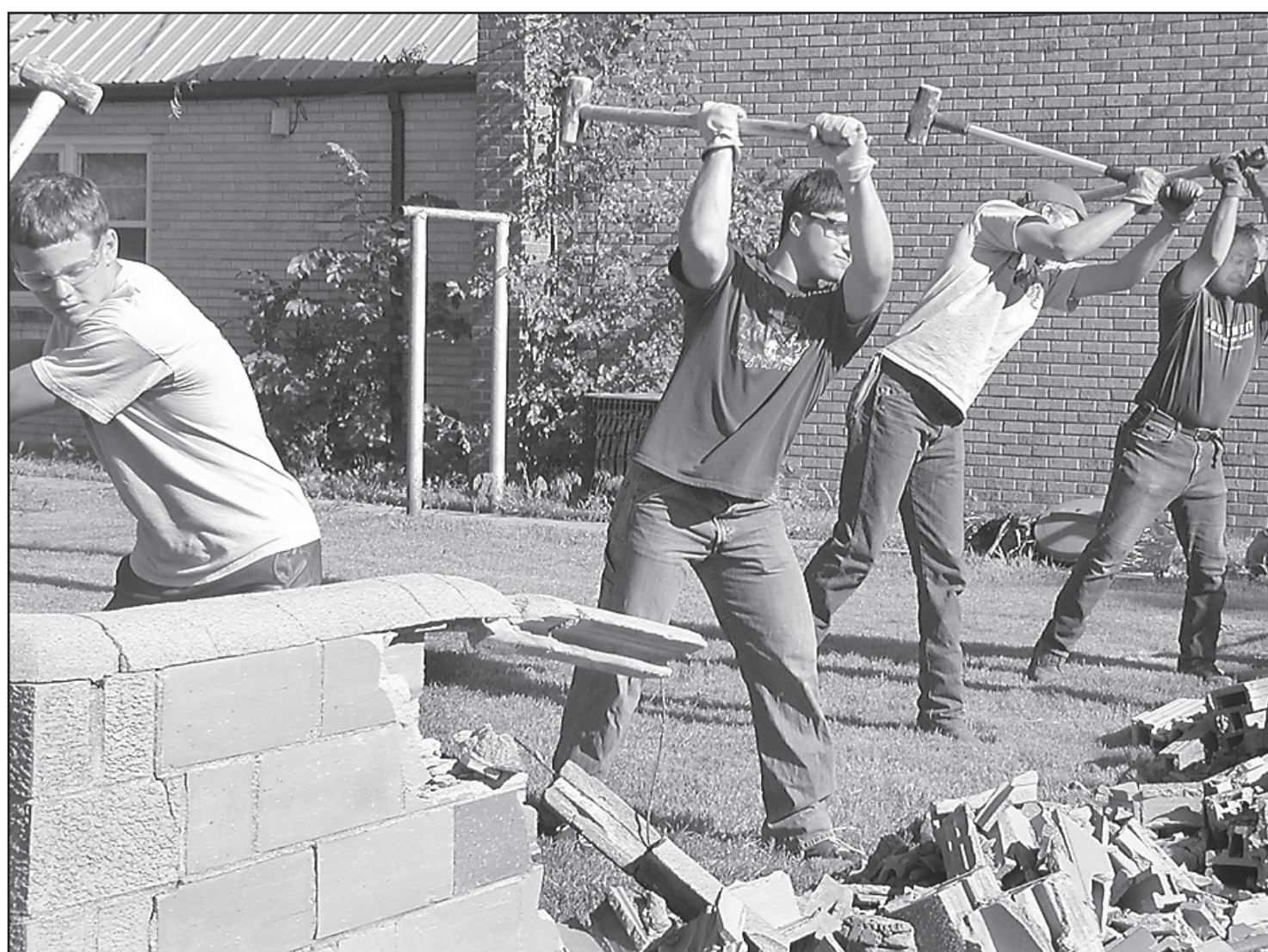
SWINGING THEIR HAMMERS almost in unison, Oberlin United Methodist youth-group members and a leader helped take down a backyard wall at the church's
