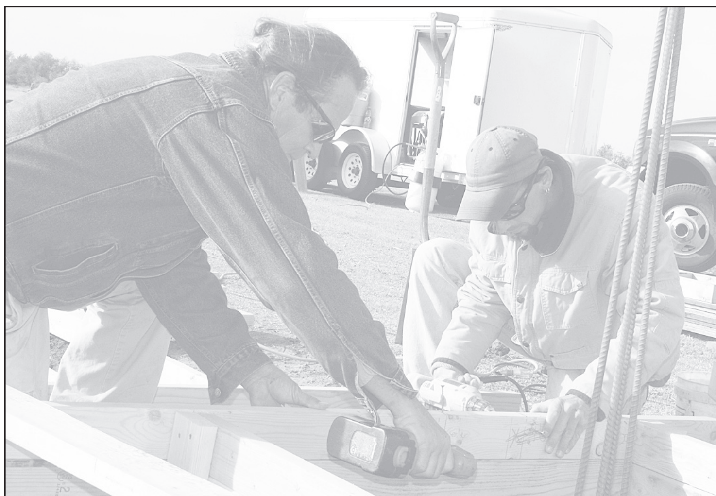
AT THE OBERLIN CEMETERY , Ken Brackhahn (left) and James Knifley set up the foundation for the new wall on the west side in preparation for the brick layers scheduled to arrive this week. — Herald staff photo by Kimberly Davis
