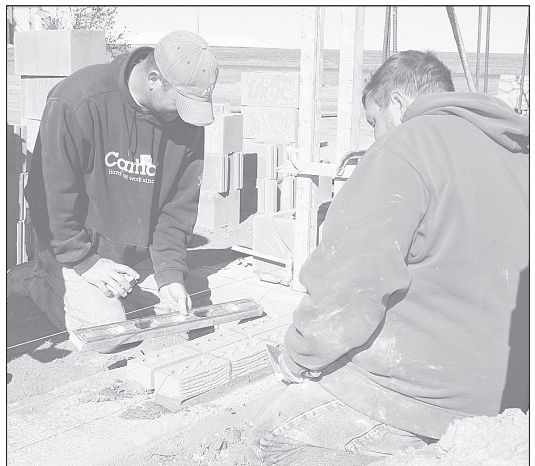
WADE NEBEN and Chris Neben placed bricks on one of the sections on the west side of Martin Ave. last week.
