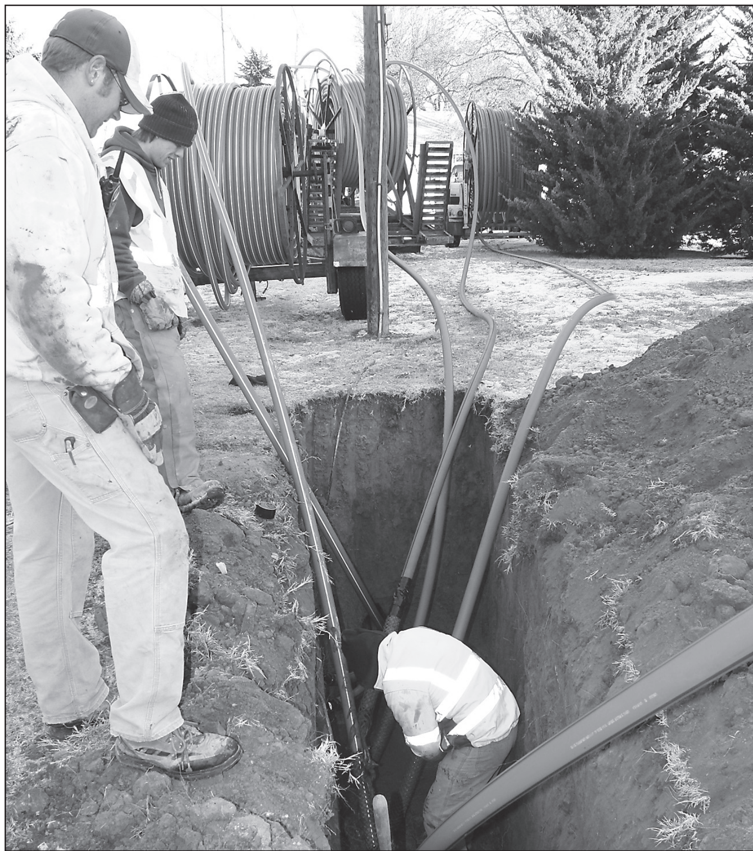
BEHIND FAITH LUTHERAN CHURCH last week, Marty Edgar (left) and Andrew Richards watched as Stan Durrant worked in a hole putting in the inter duct for fiber optic lines for Nex-Tech Communications, an affiliate of Rural Telephone. The men work for Johnson Construction of Weyauwega, Wis. — Herald staff photo by Kimberly Davis
