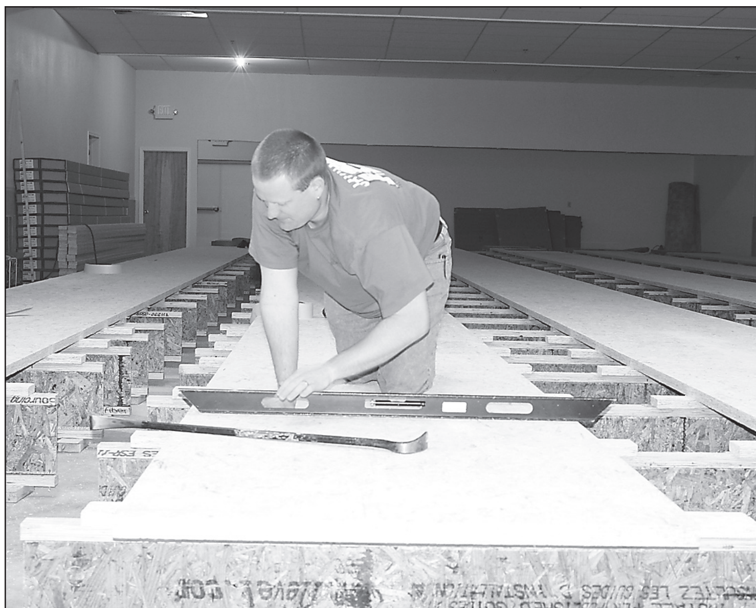
AT THE BOWLING ALLEY, Bryan Selters, with Jayhawk Bowling, worked on getting the new lanes in on Monday afternoon.
