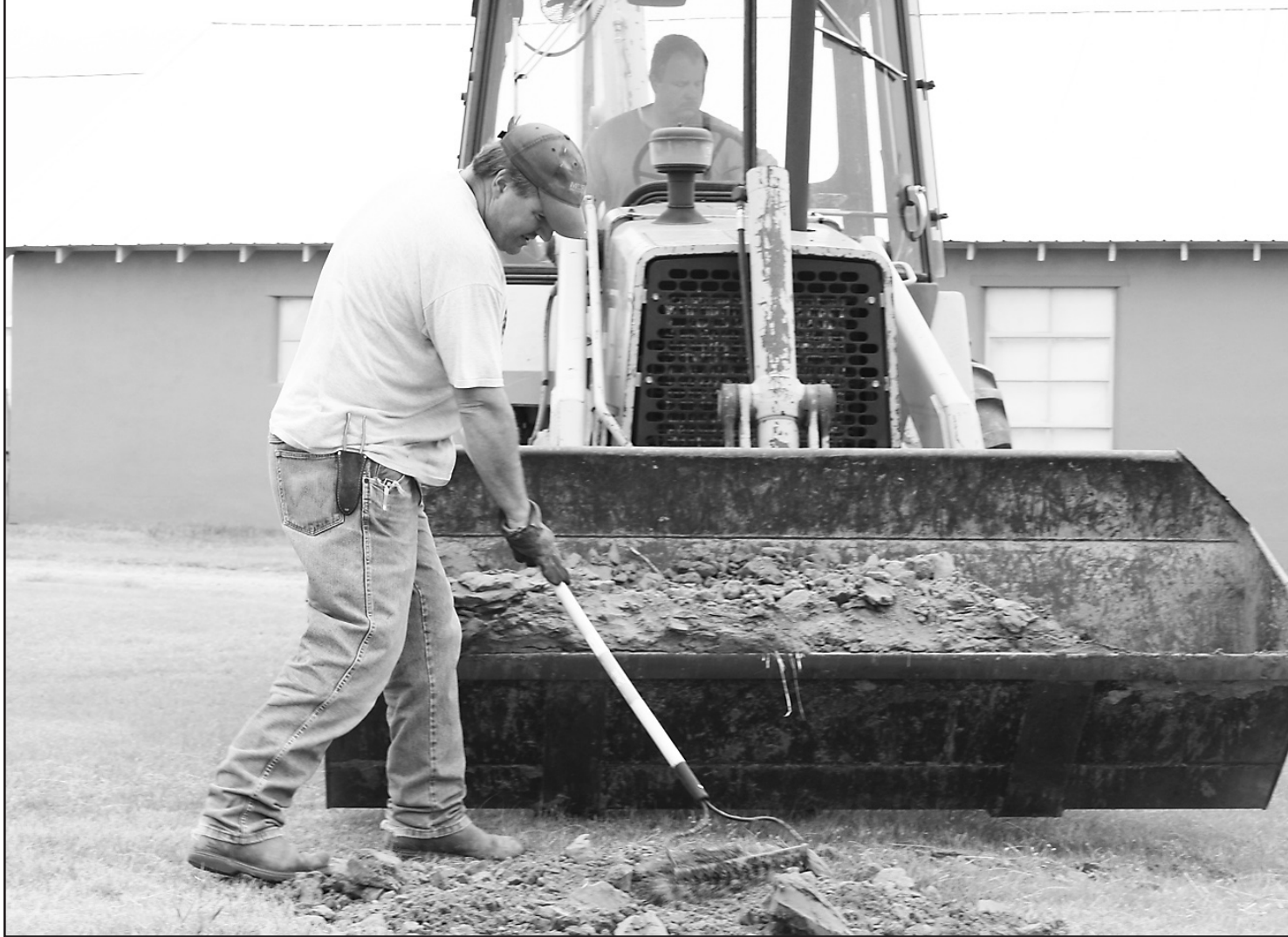
AT THE DECATUR COUNTY FAIRGROUND on Monday, Seth Lohofener used a rake to spread dirt evenly over a hole while operator Justin Scott sat in the front-end
