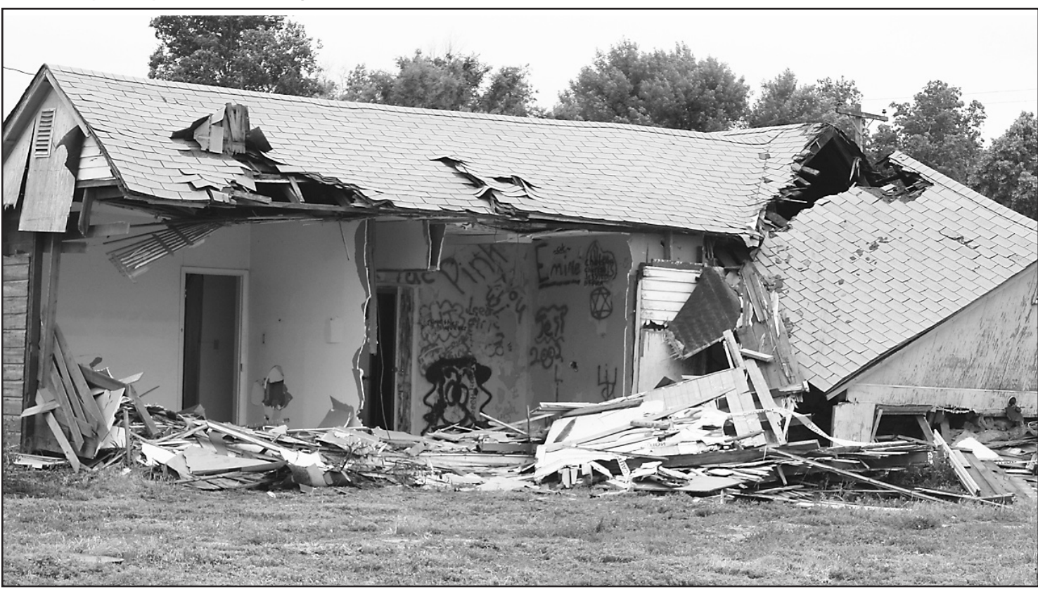
NEW OWNERS Jeff and Elizabeth Sprenkle have started tearing down the blue house at 302 W. Hall. The home, formerly owned by Nolan and Bobbi Jo Johnson, had been in the condemnation process by the city. The Sprenkles sent
