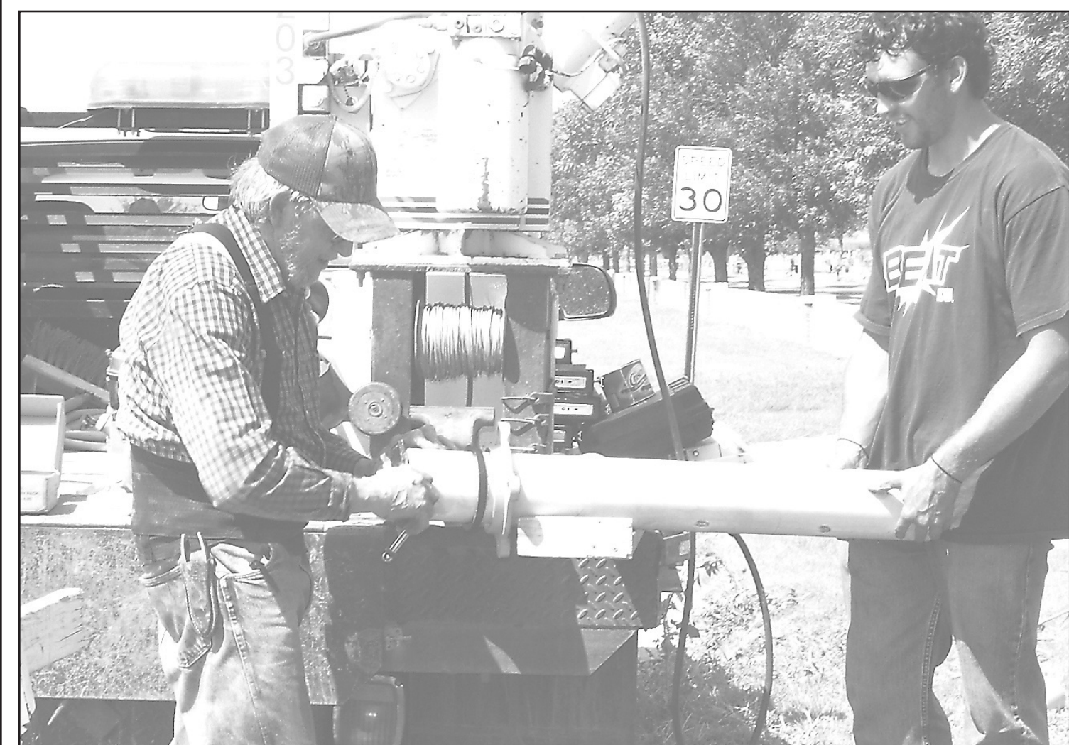
ON THE SOUTH SIDE of the city cemetery Thursday afternoon, Willard Perrin and Derek Chambers of the city water crew replaced a valve and pipe that had gone bad some time ago. — Herald staff photo by Kimberly Davis
