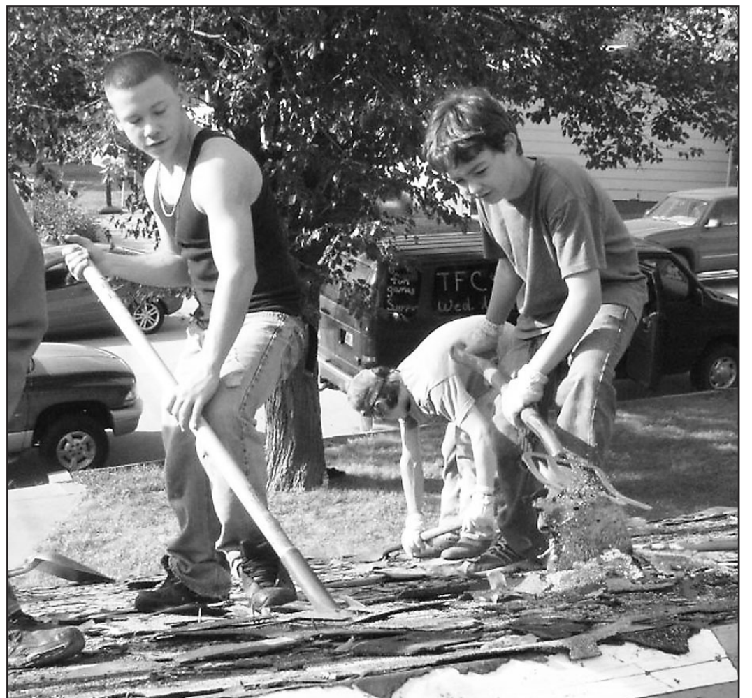
TOOLS IN THEIR HANDS, Triston Sepeda and Daniel Lerew helped tear off the old roof.
