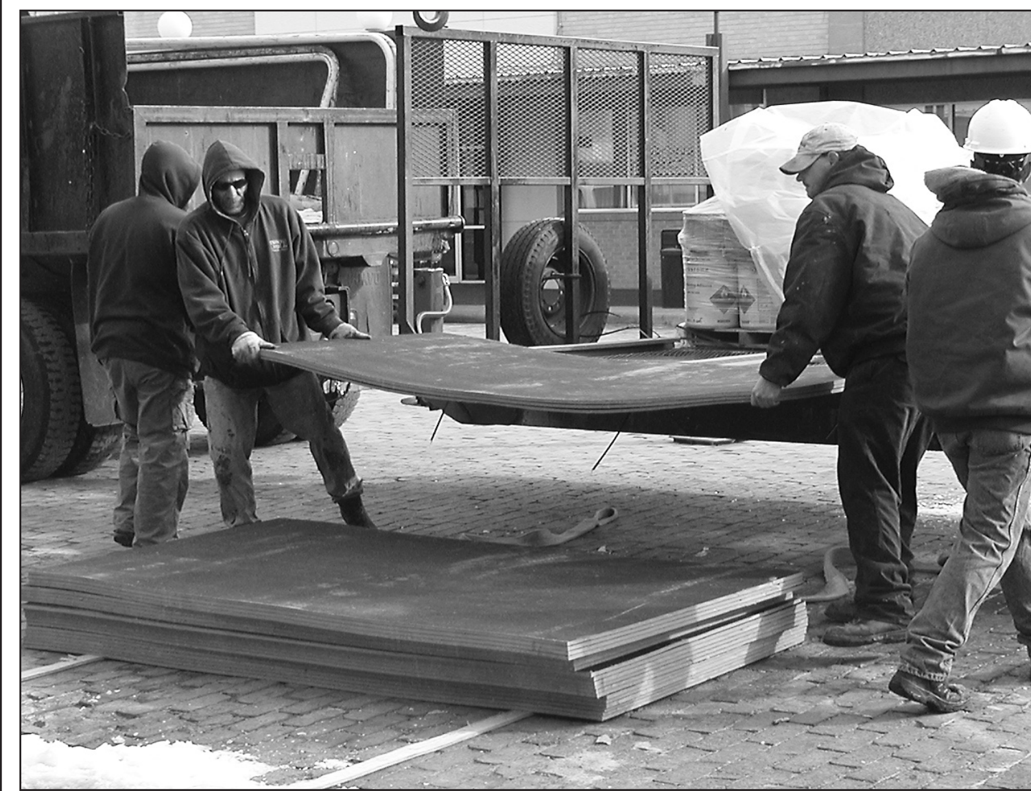
WORKMEN MOVED ROOFING material onto straps and tall crane drew several onlookers Monday morning. — Herald staff photo by Cynthia Haynes
