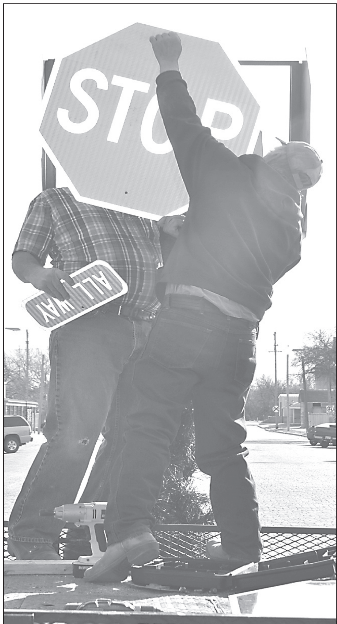
IT PROBABLY SHOULD have been a stop light, but Ron Solko could only replace this old stop sign at Hall Street and Penn Avenue with a shiny new one. Melvin Martin (behind the sign) assisted with the project. The stop lights were taken down when the city renewed the sidewalks around them, and now await some needed parts.
