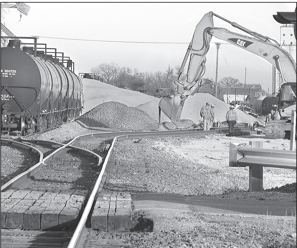
RAILROAD EMPLOYEES REROUTED the track around a collapsed elevator in Oakley by pulling it to one side with a back hoe (above), then connecting the two ends with prebuilt track panels. After as much of the original track as possible had been pulled onto the new alignment, workers bolted in additional sections of rail to form a detour around the pile of spilled corn.
