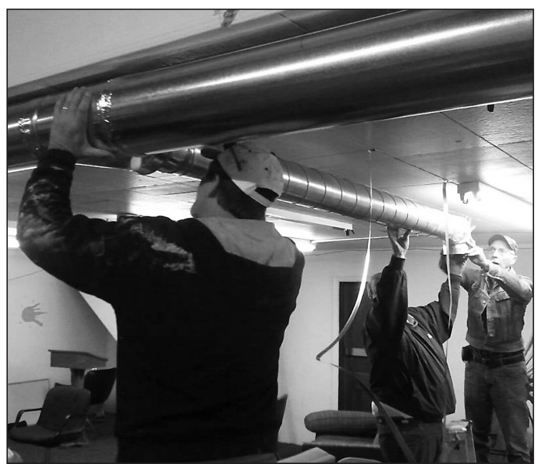
COMPLETING A SERVICE PROJECT at the Oberlin Teens for Christ building last week were several members of the McCook Evangelical Free Church, including Larry Ganje (right) of Oberlin. The church members supplied material and labor to extend existing duct work for the building.
