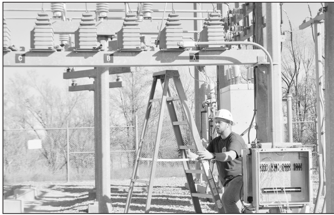
SQUINTING IN THE AFTERNOON SUN, Justin Byarlay of Mid-States Energy Works out of Salina surveyed part of the city's main electrical substation during repairs in October. --Herald staff photo by Stephanie DeCamp
