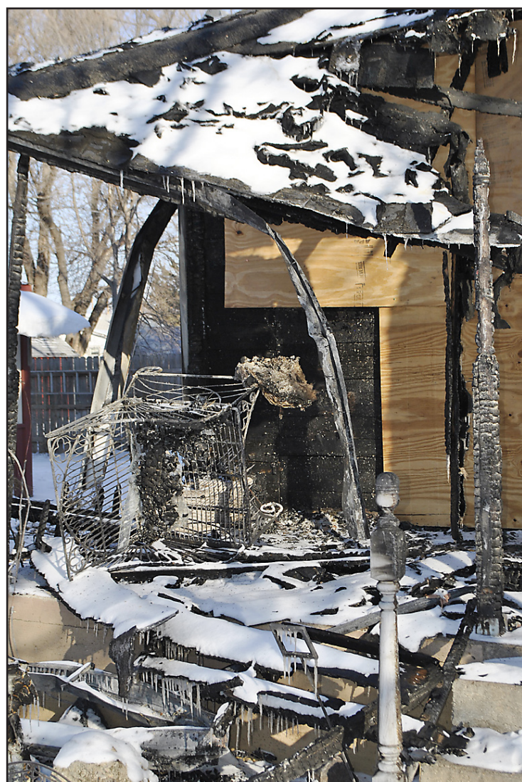
A FIRE at Laurie Milnes' home on East Commercial Street started from a short in a pinched wire and quickly spread through the old Victorian home, said Fire Chief Bill Cathcart. The house was assessed to be a total loss.
