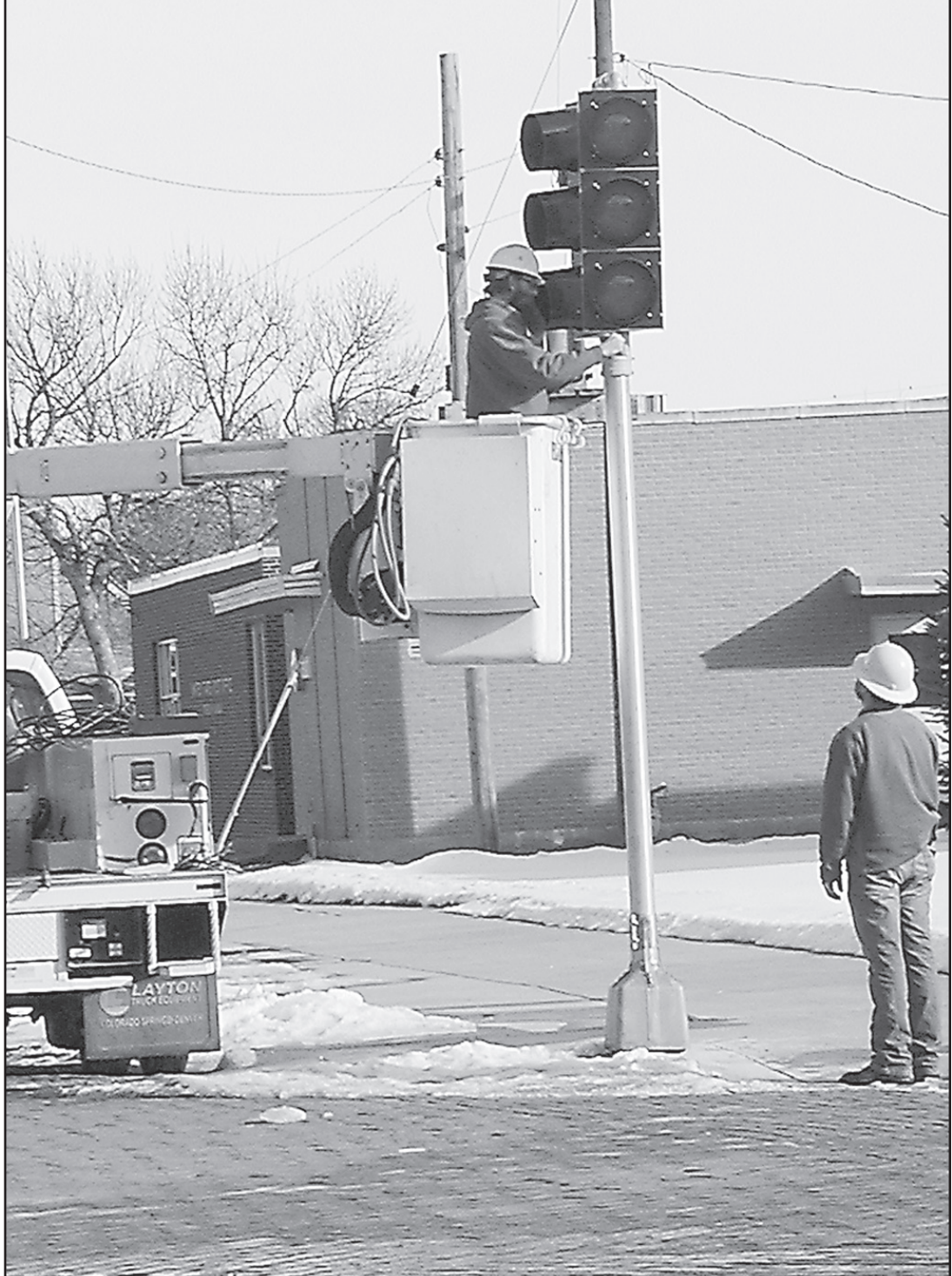
REPAIRING ONE OF THE FOUR stoplights at Penn Avenue and Hall Street, city workers David Perrin (up in the air) and Logan Fortin got the lights into blink mode Friday. The four-way stop sign, which has been decorating the middle of the intersection (and at Christmas was decorated), has now been put away. — Herald staff photo by Cynthia Haynes
