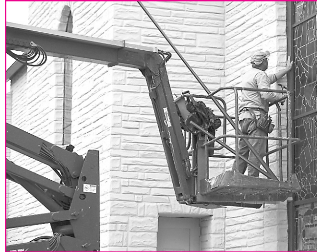
FINLEY CONSTRUCTION OF ATWOOD finished covering all the windows of St. Mary's Catholic Church in Herndon with Plexiglas. The church hopes that this will prevent further paint damage to the interior walls. Workers were Rod Carroll, Chris Lamb and Doug Merz.
